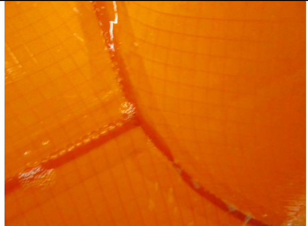
This image shows a slow leak in one of the cross seams.
